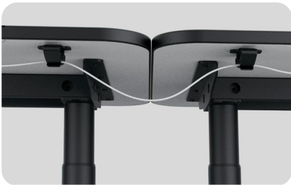
Training Room, managing cables from desk to desk.
